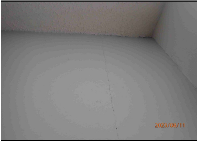
Photograph 25 - P8110231 - vertical hairline crack in unit 17.
