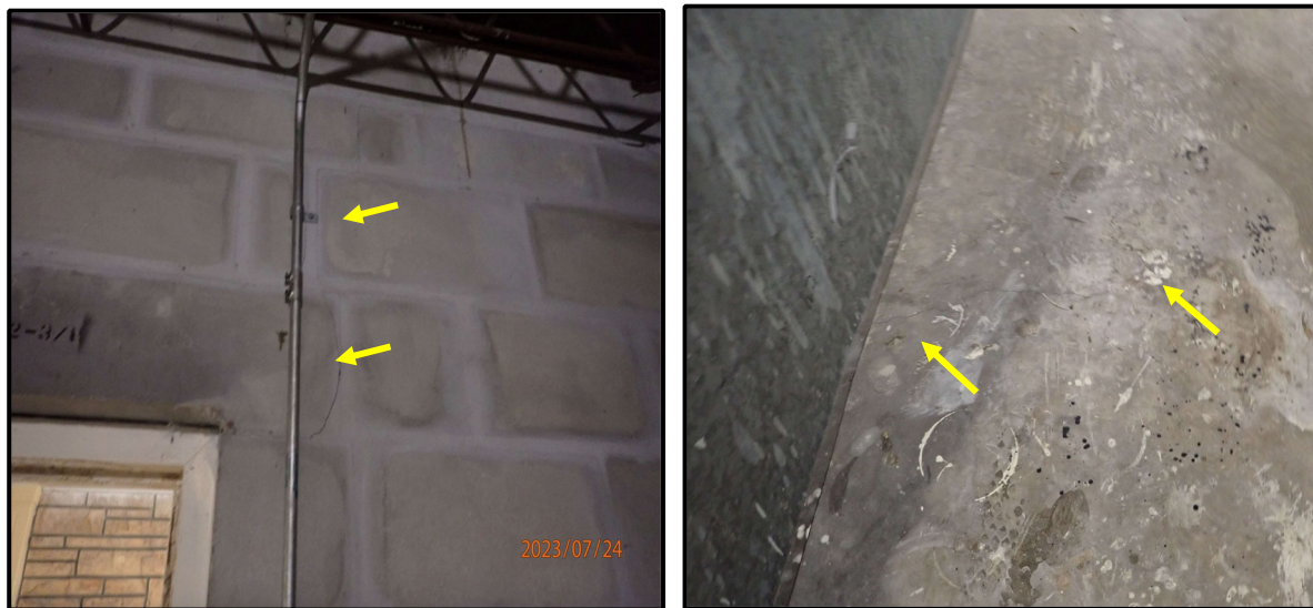
Figure 9. Representative photographs of cracks on CMU walls and concrete slabs at common rooms in Core building.
