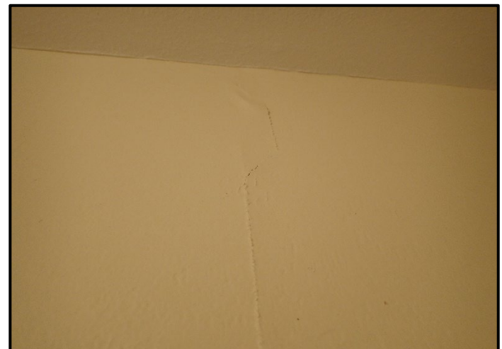
Photograph 24 - P8171774 - vertical hairline crack in unit 6.
