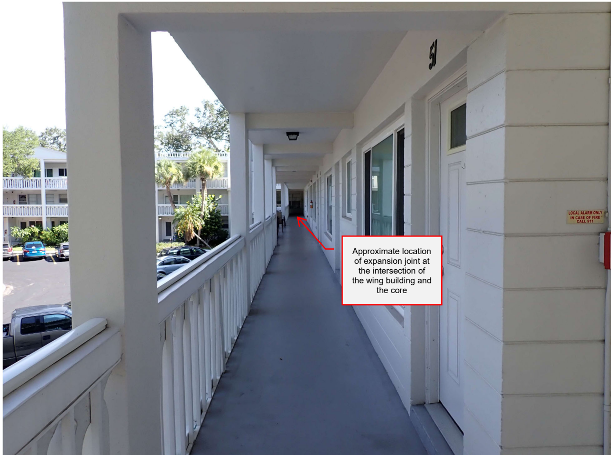
Figure 6. Representative approximate location of expansion joint at wing/core intersection in representative building.
