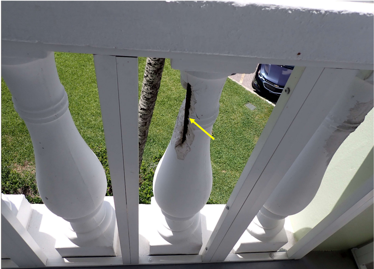
Figure 10. Representative photograph of cracking of decorative railing
