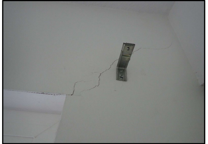
Photograph 26 - P8100069 - vertical hairline crack in unit 53.
